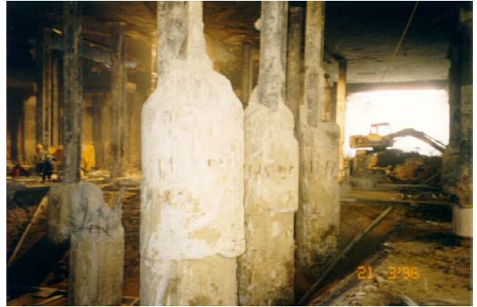
Fig. 6 The photograph illustrates the pile size changes caused by difference in diameter of temporary casing and auger used in pile construction.
