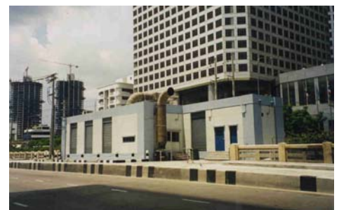
Sathorn pump station.
