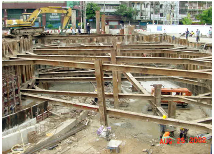
Excavation with braced sheet pile for construction of base slab and retaining walls.
