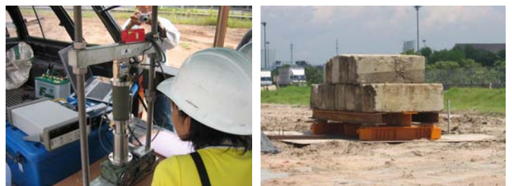
Quality control tests— Column extraction, UCS test on core samples and static load test.
