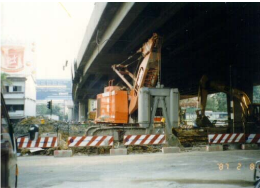
Diaphragm wall panel excavation with modified grab crane under the existing expressway.
