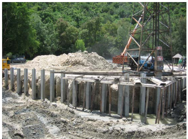
Installation of concrete facing walls for boat berth and ramp by other — soil retained by soil-cement columns.
